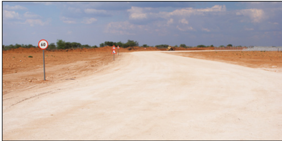
The new bypass gravel road that motorists will use to access the Letlhakane Mine lease area
